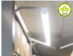
AUTOMATIC OVERHEAD AISLE LIGHTING
