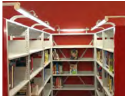
LED AISLE LIGHTING
